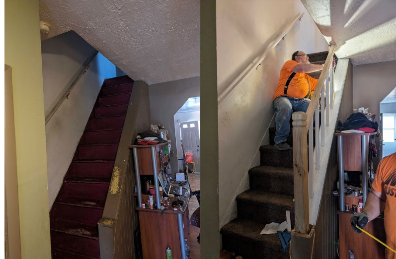
Figure 13: Before and after repairs at one of the homes served by Southeast CDC.
